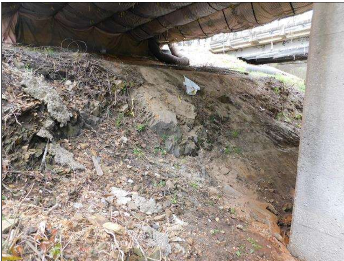
32' x 10' x 4' deep erosion on South streambank
