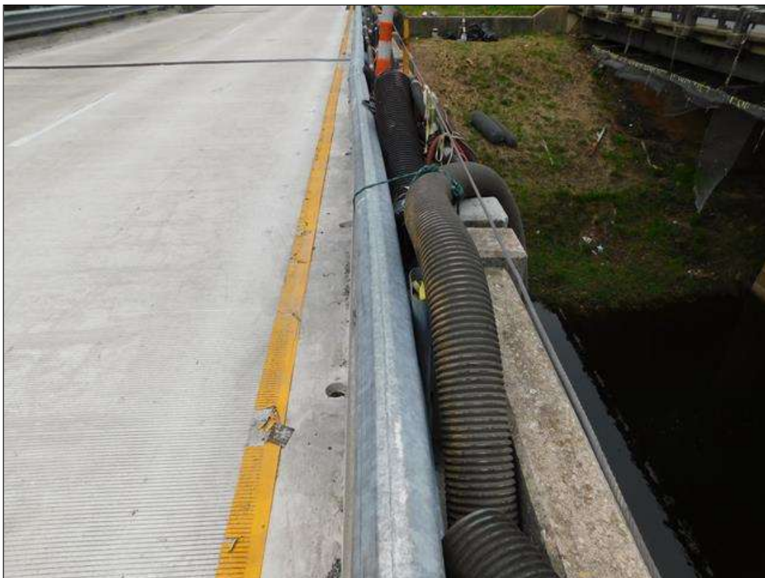
Span 2 Left Bridge Rail: 20' impact damage with 2" deflection to the West on metal rail
