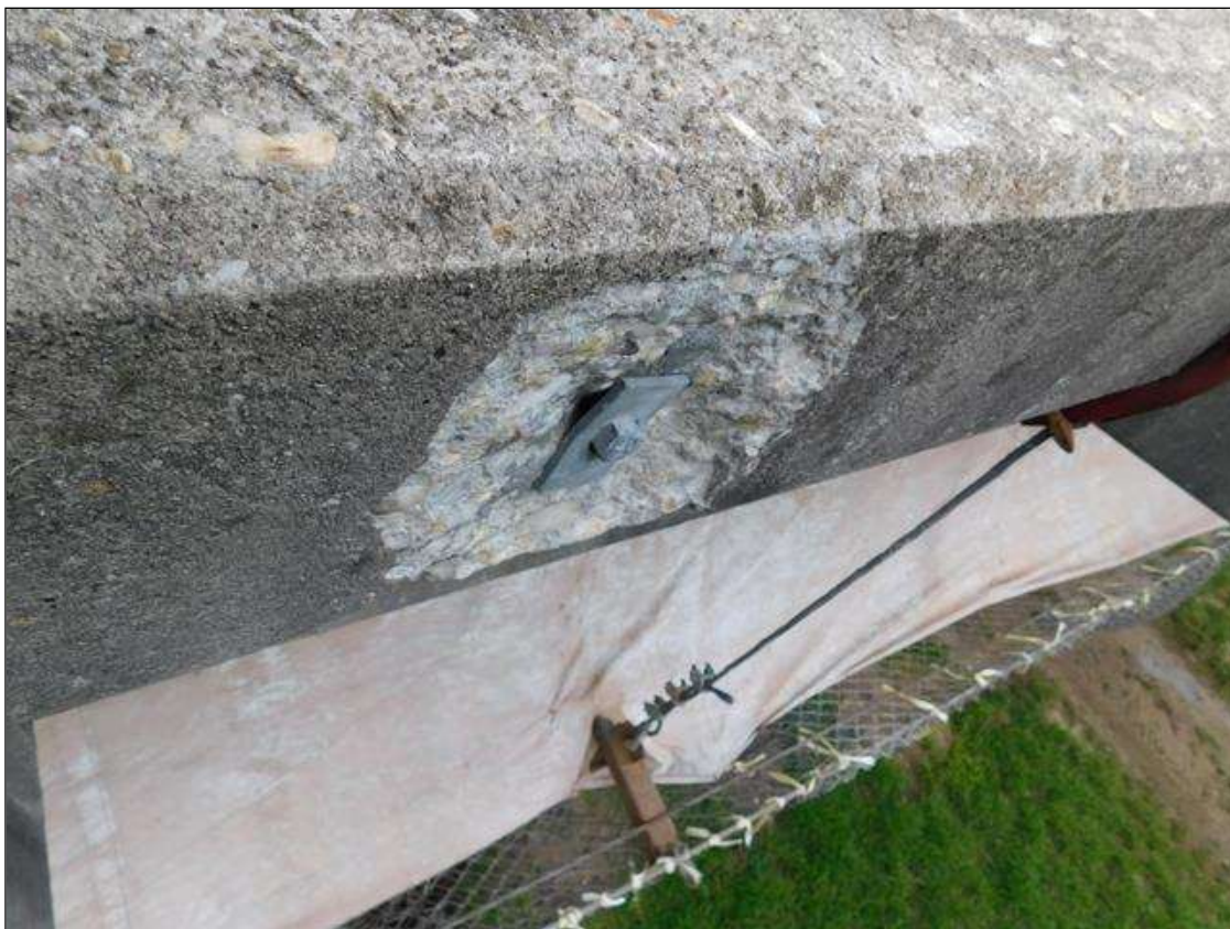
Span 3 Right Bridge Rail: (3) up to 9" x 9" x 1" deep spalls on outside face of concrete rail
