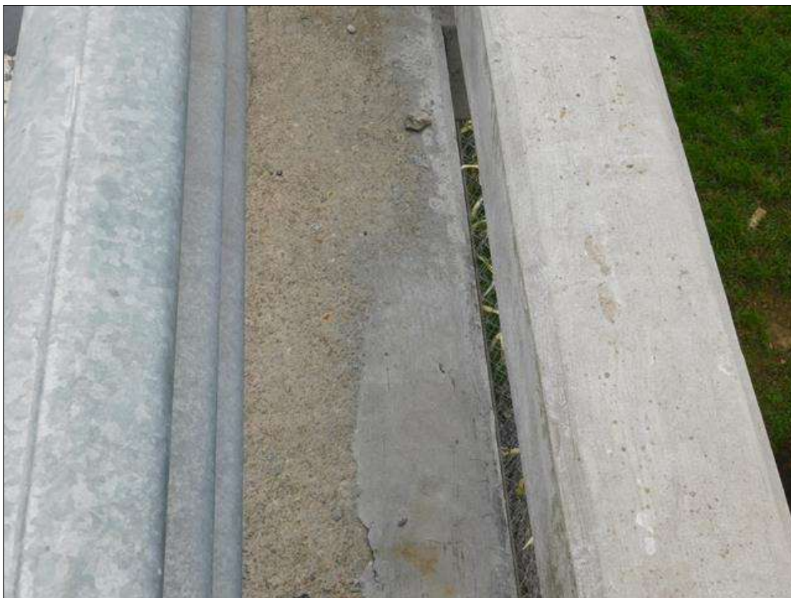
Span 2 Right Bridge Rail: 36" x 9" area of patch with hairline map cracking on curb near Bent 2
