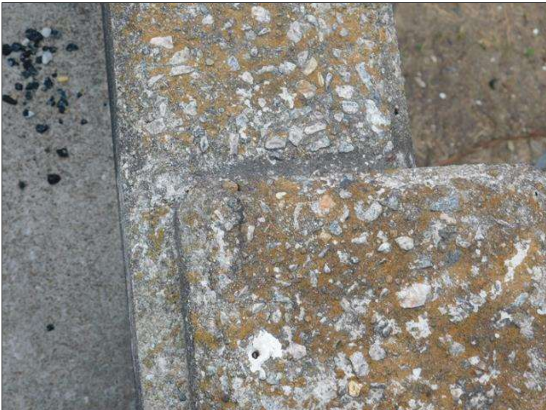
Span 1 Right Bridge Rail: 3" hairline longitudinal crack on Post 3
