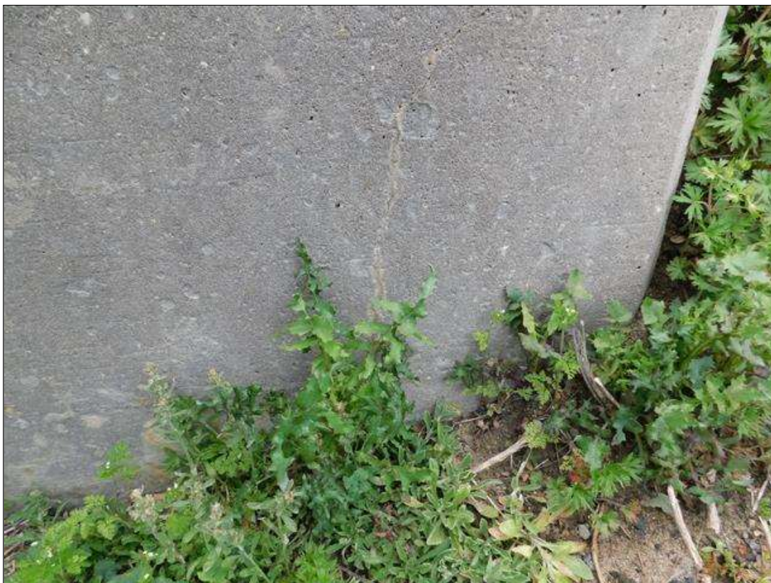
(2) up to 28" hairline vertical cracks with efflorescence on Northwest wingwall
