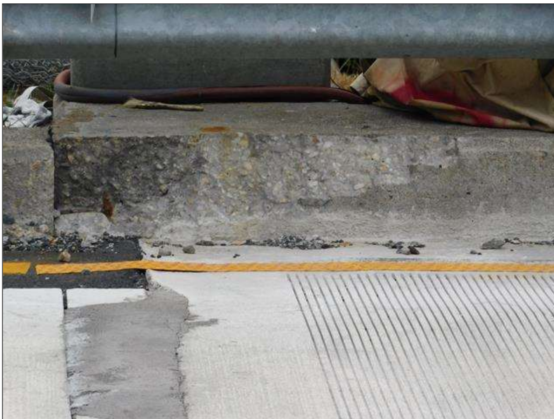
Span 1 Left Bridge Rail: 35" x 9" x 2" deep spall with exposed rebar on curb at End Bent 1
