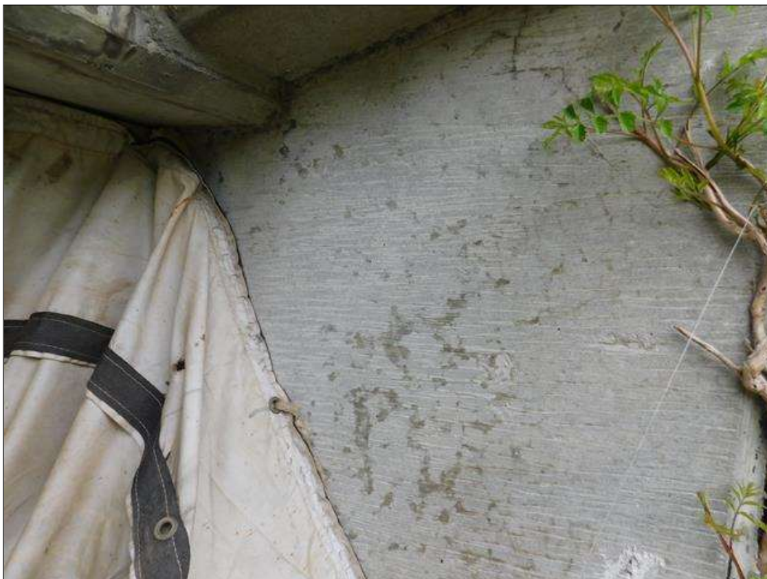
End Bent 2 Abutment/Backwall: 2' x 3' area of hairline map cracking at East end (West end similar)
