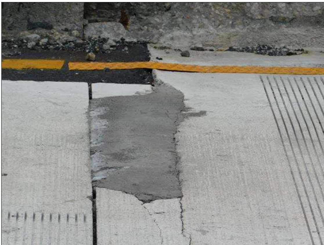
Span 1 Deck: 4" x 4' area of patch with hairline transverse crack in West lane at End Bent 1
