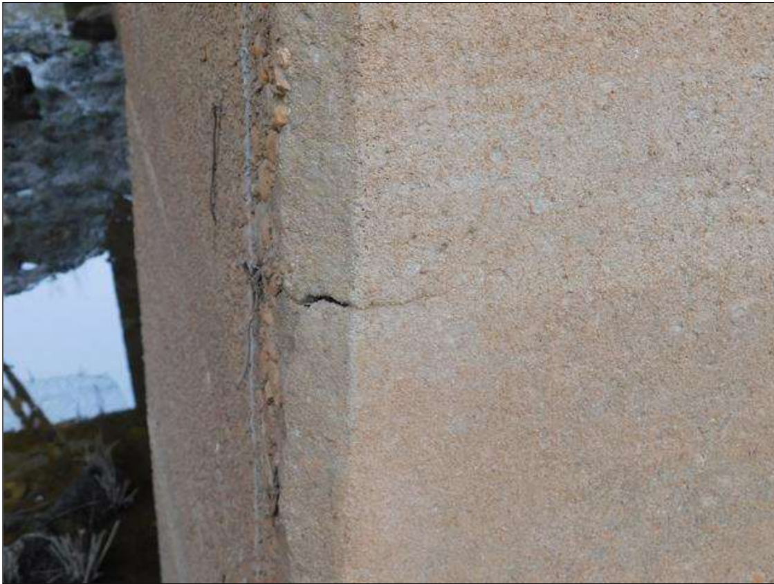
Bent 3 Pile 1: 6" up to 1/16" horizontal crack on West face
