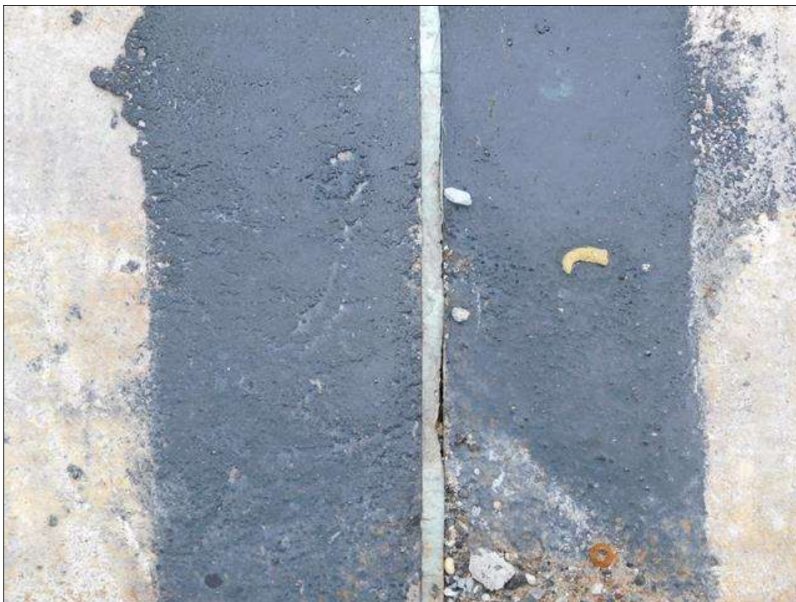
Expansion Joint: 7" x 1/2" deep detached joint material in East lane
