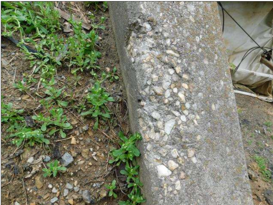
17" x 6" x 1 1/2" deep spall on Southeast wingwall
