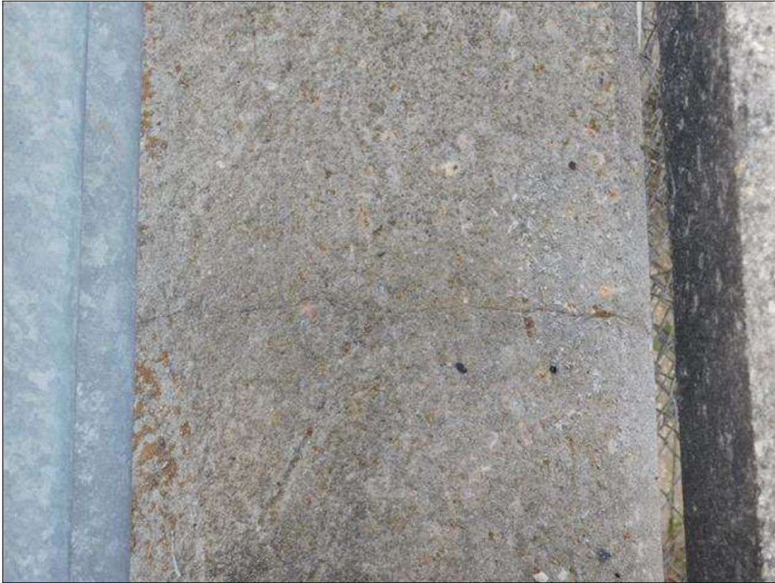
Span 4 Right Bridge Rail: (5) hairline vertical and transverse cracks on concrete curb and rail
