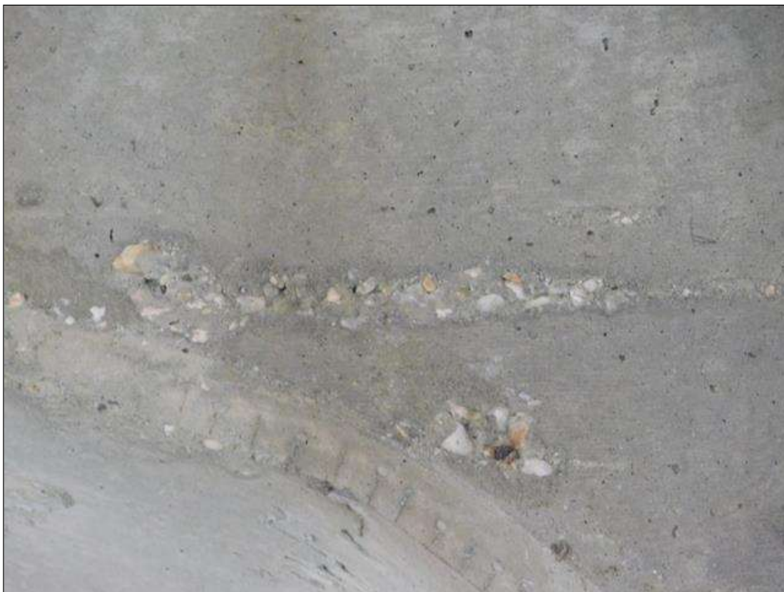
Bent 2 Pile 2: 2" x 10" x 1/2" deep spall on East corbel on Span 3 face
