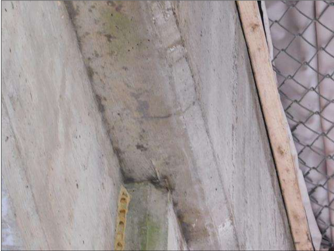
Bent 2 Cap 1: (13) up to 5" hairline longitudinal cracks on bottom of cap between Columns 1 and 2
