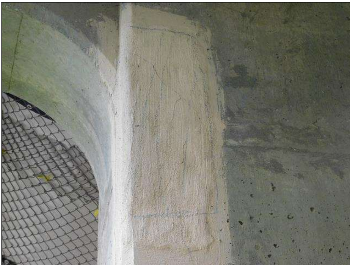
Bent 3 Pile 1: 28" x 11" area of patch with hairline vertical and diagonal crack on Span 3 face
