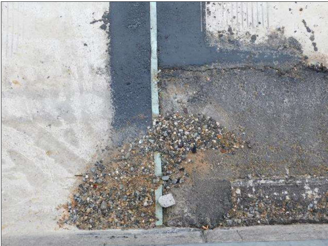
Expansion Joint: 2' dirt and debris in East gutter
