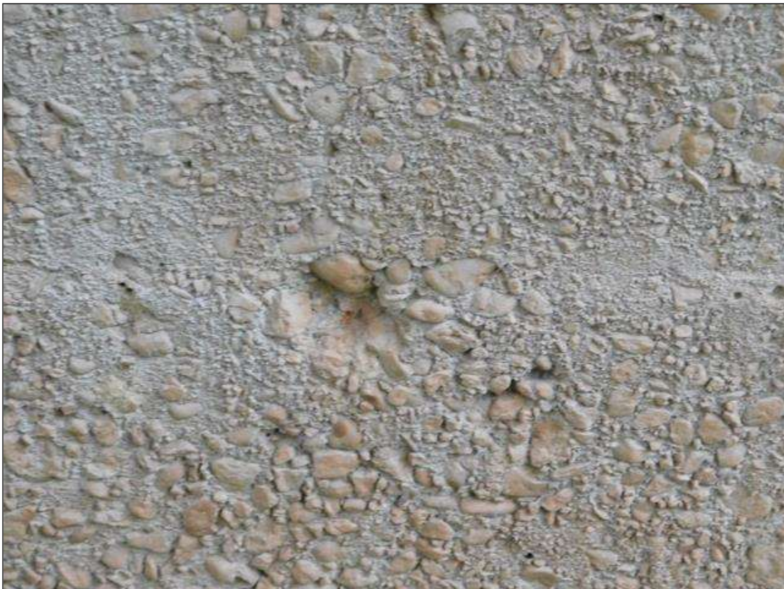
Bent 3 Pile 2: (3) up to 2" x 2" x 1/2" deep spalls on Span 3 face
