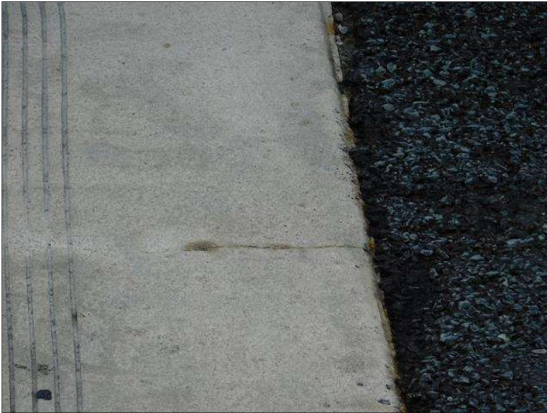
Approach 2: 1 square foot hairline longitudinal crack in East lane
