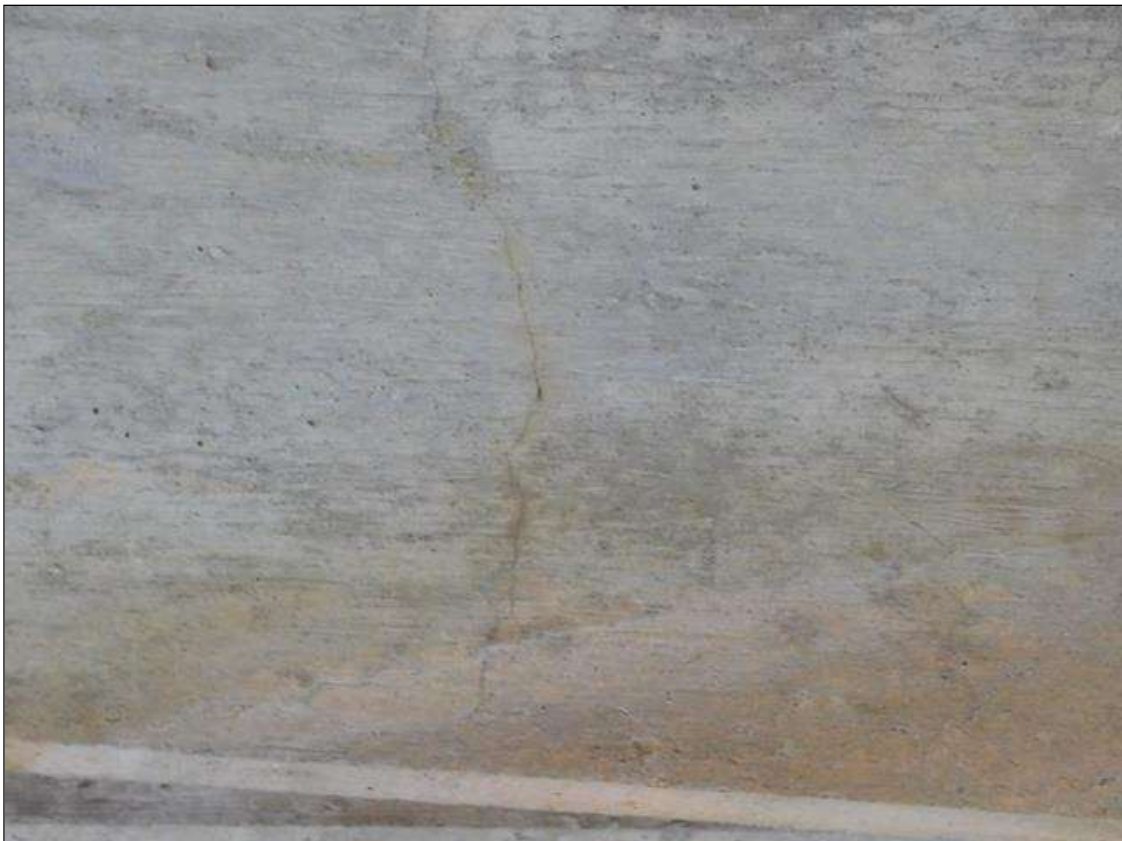
Bent 2 Cap 1: (3) up to 20" hairline longitudinal cracks on bottom of corbel between Columns 1 and 2
