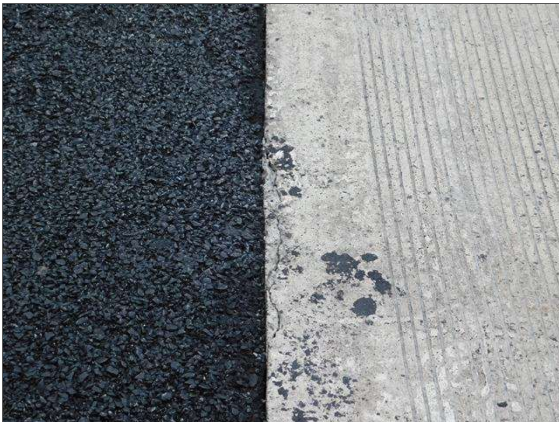
Approach 1: 3 square feet up to 1/16" transverse crack in East lane at South end
