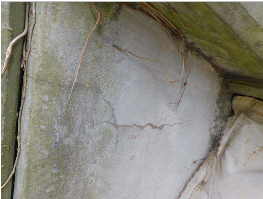
End Bent 1 Abutment/Backwall: 27" x 11" area of hairline vertical and horizontal cracks at East end
