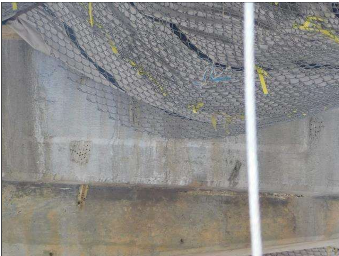
Bent 2 Cap 1: 6' x 2' area of sound patch on Span 2 face, 8' from East end
