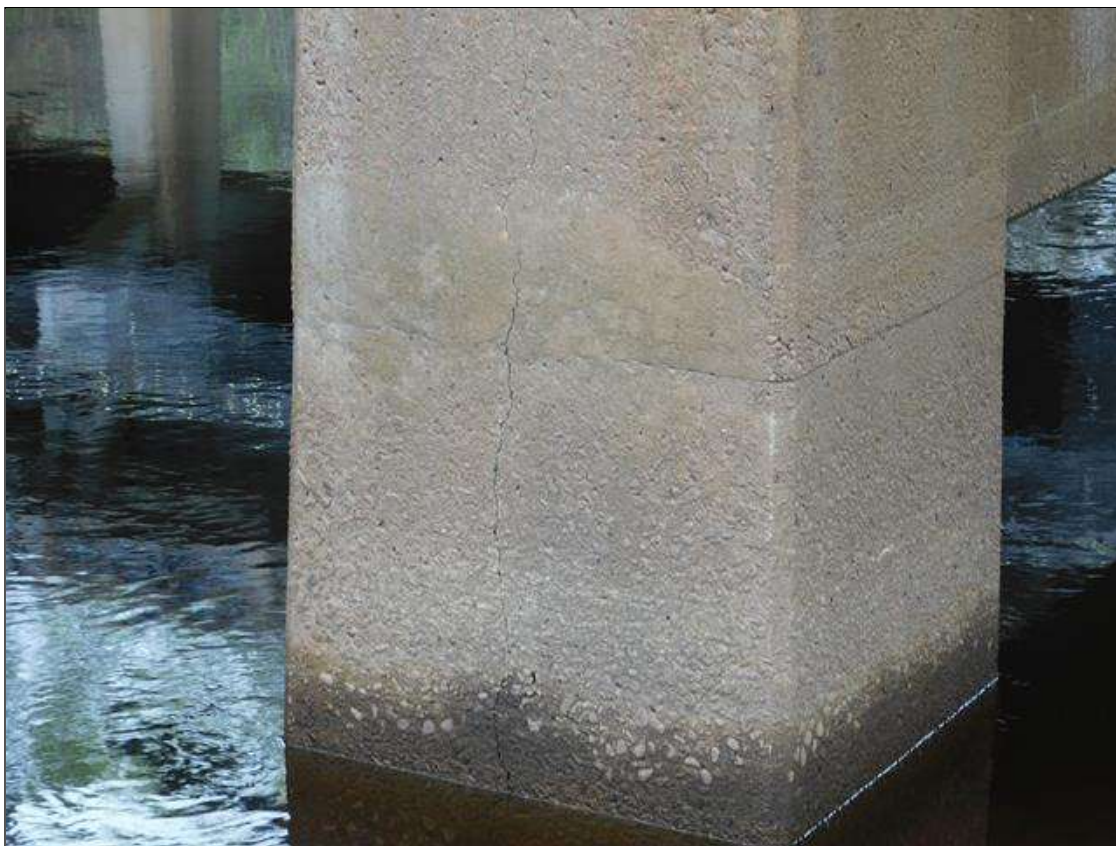
Bent 2 Pile 2: 46" up to 1/16" vertical crack on East face (Span 3 face similar)
