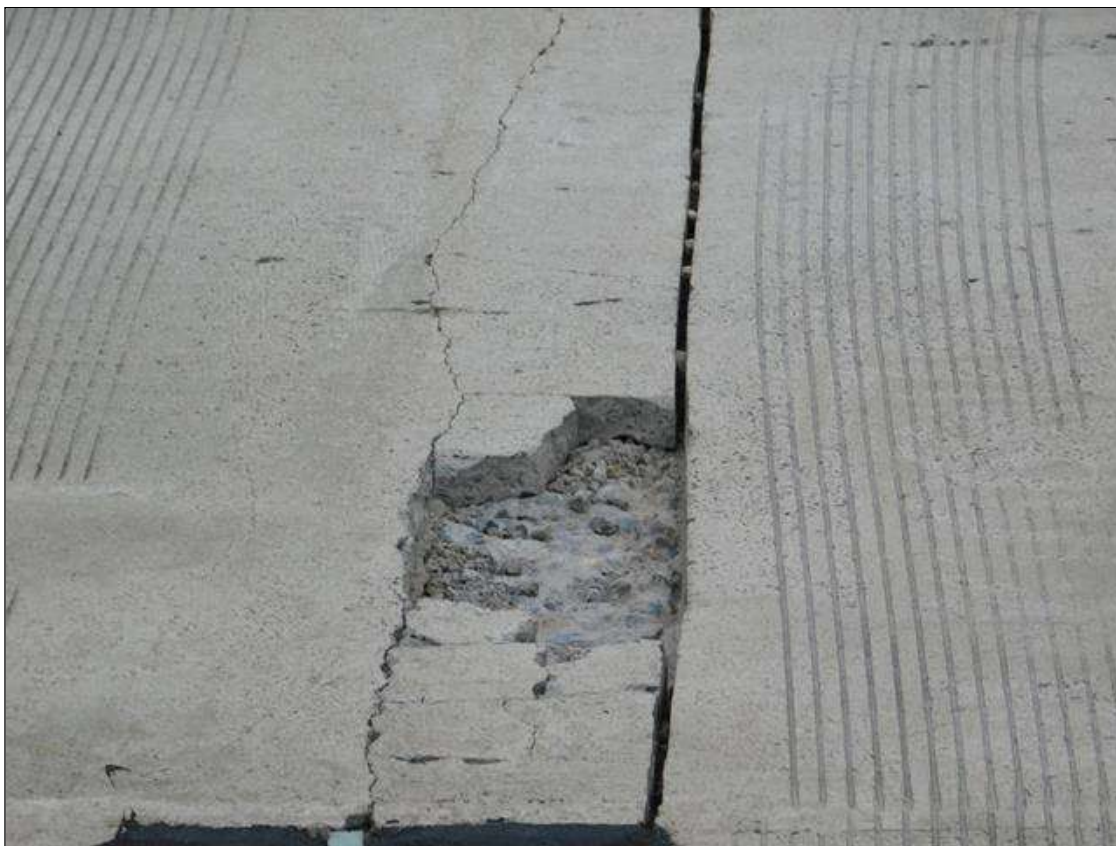
Expansion Joint: 30" x 6" x 2" spall along joint in West lane
